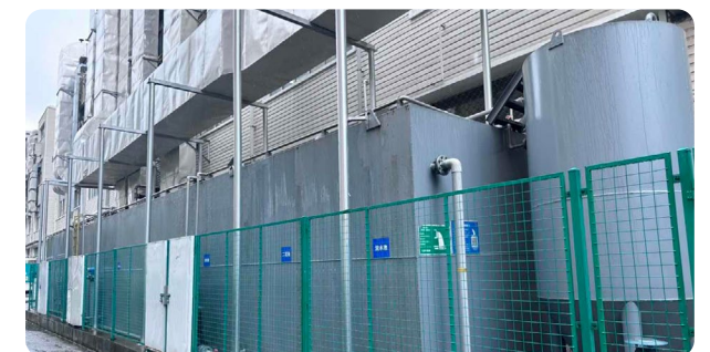
Integrated Sewage Treatment Unit
